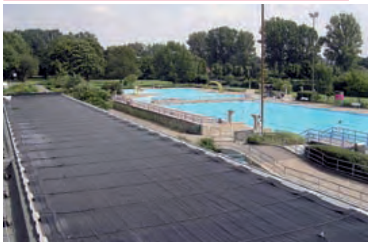
Solar thermal plant at Lister Bad open-air pool
