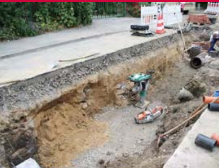
Typical road fretting with rubble in the substructure
