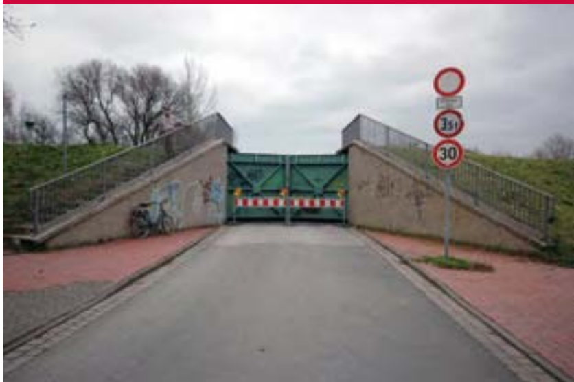
Closed dike gate in Ricklingen
