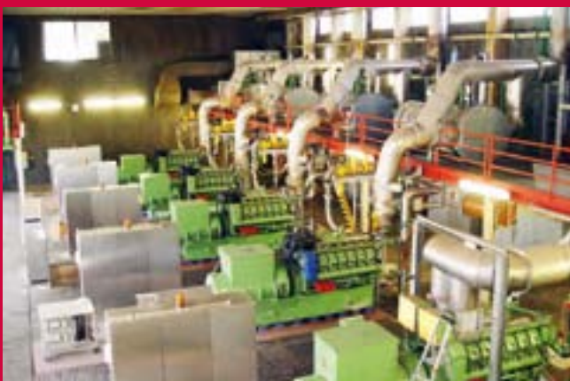
CHP Plant in Herrenhausen sewage treatment plant
