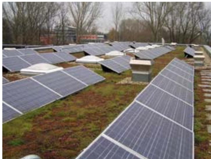
Combination – roof greening and photovoltaic installation Werkhof Stammestraße
